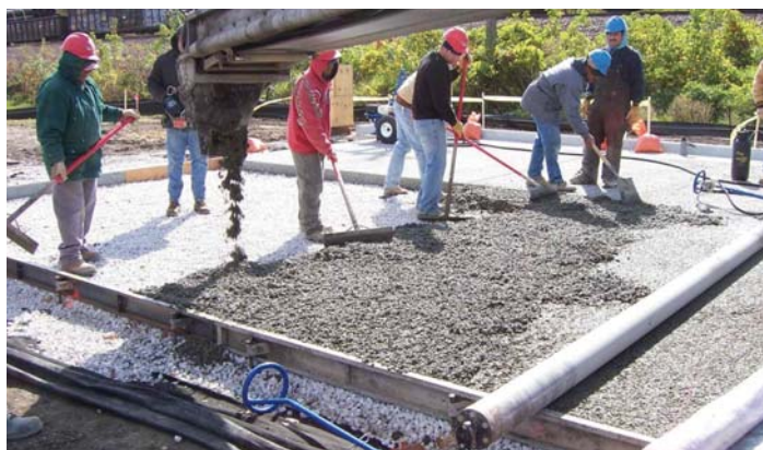
Placement of pervious concrete pavement (courtesy of John Kevern, University of Missouri-Kansas City)
