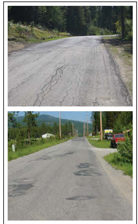
Figure 1. Deteriorated asphalt pavements that are candidates for full-depth reclamation with cement
