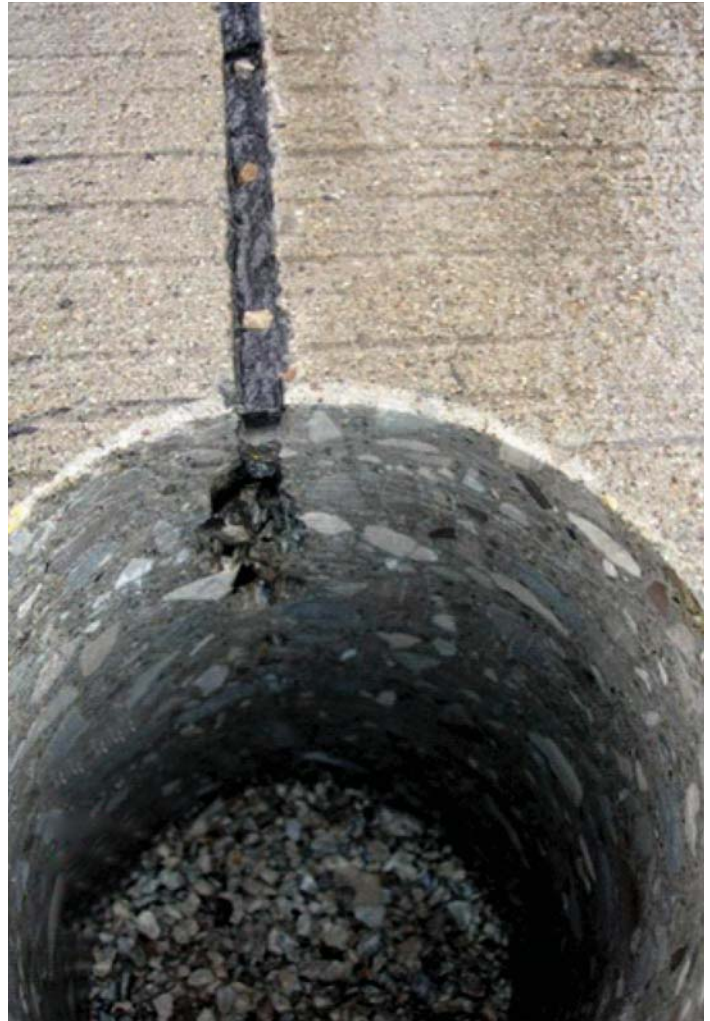
Figure 5. Example of damage occurring in a slab that has not cracked out
